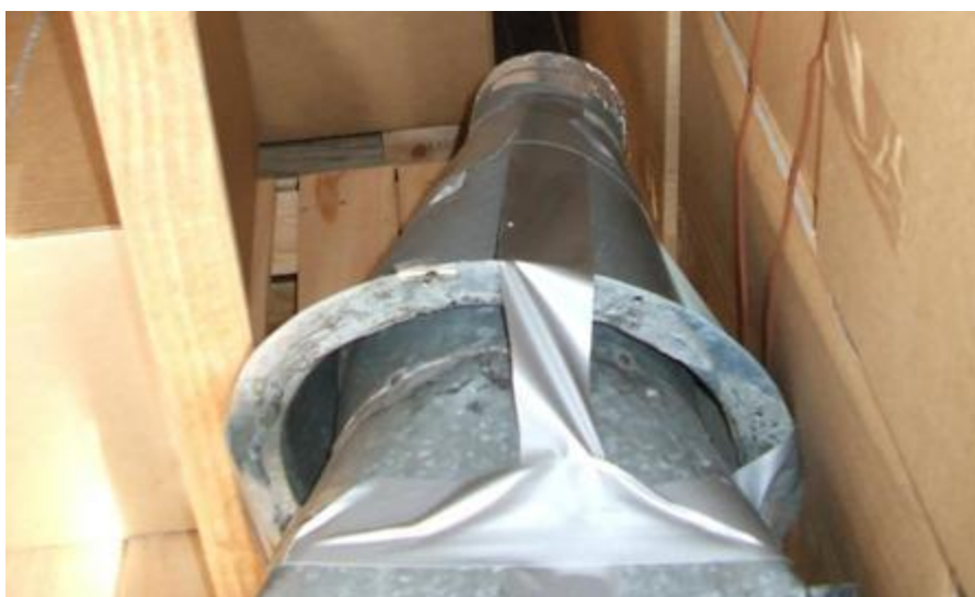
Fig. 3.10: The auxiliary fan fitted with outlet cone.
