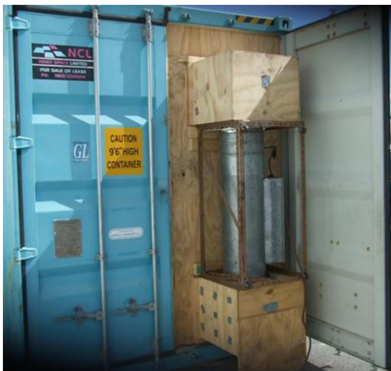
Figure 3.8: The heating unit fitted to the container door way.
